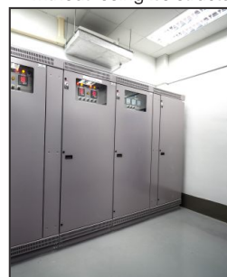
Fireproof storage room for solar batteries and inverters
